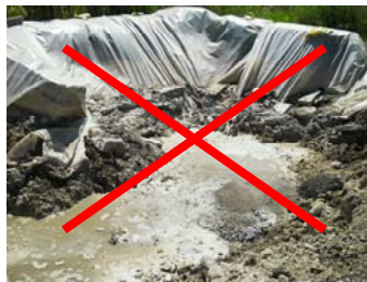
Failed washout pit
