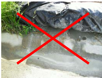
Leaking washout pit
