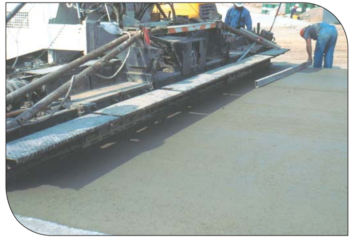
A smooth, durable RCC pavement can be achieved that will provide excellent performance for many years.
