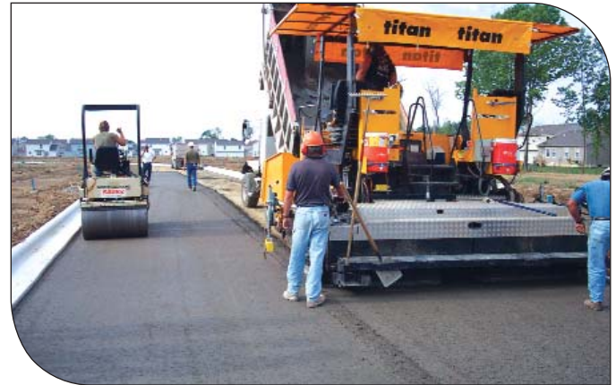
Constructing city streets in Columbus, OH using RCC is quick and convenient. Residents can drive on the RCC base soon after final rolling.
