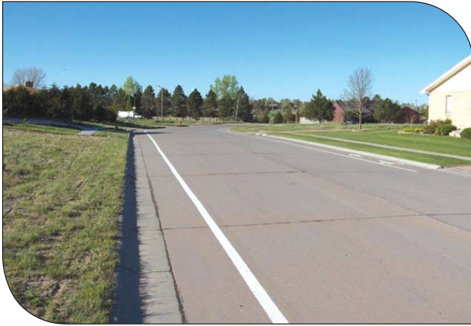
Unsurfaced RCC street in Alliance, NB shows little sign of wear 11 years after construction.
