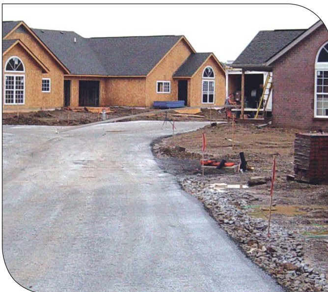
RCC placed during site work serves as a working surface. With a thin overlay, it becomes a residential street once construction is complete.
