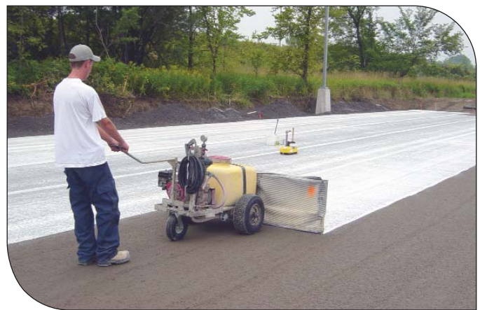
A key to long term performance is adequate curing. Water or concrete curing compounds are typically used.
